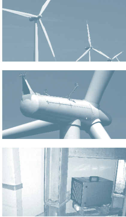
Installation inside wind turbine tower.
